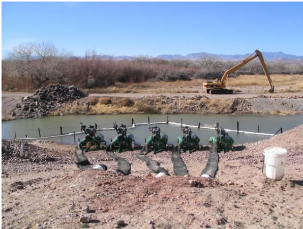
Figure 3.18. Low Flow Conveyance Channel Pumps
